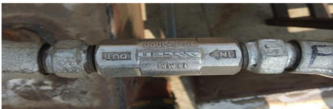
Fig.2.1.5: Flange and NRV
